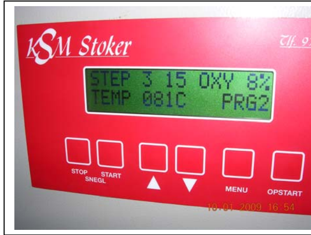
Programmable Boiler Control
