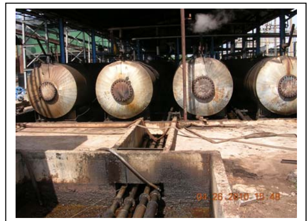
The sterilizers blow down pipes and the canal from the sterilizers leading to the pit.
