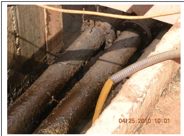
The effluent from the test unit is sent back into the POME collection pit. The pipes seen are from sterilizer blow down and the canal below the pipes is leading POME from underneath and around the sterilizers to the pit.
